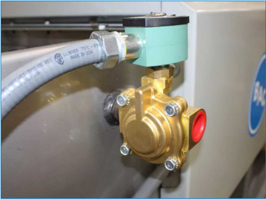
Drain solenoid valve
