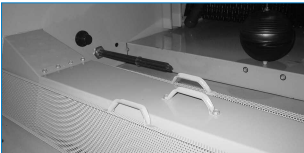
Cold water basin and basin strainer
